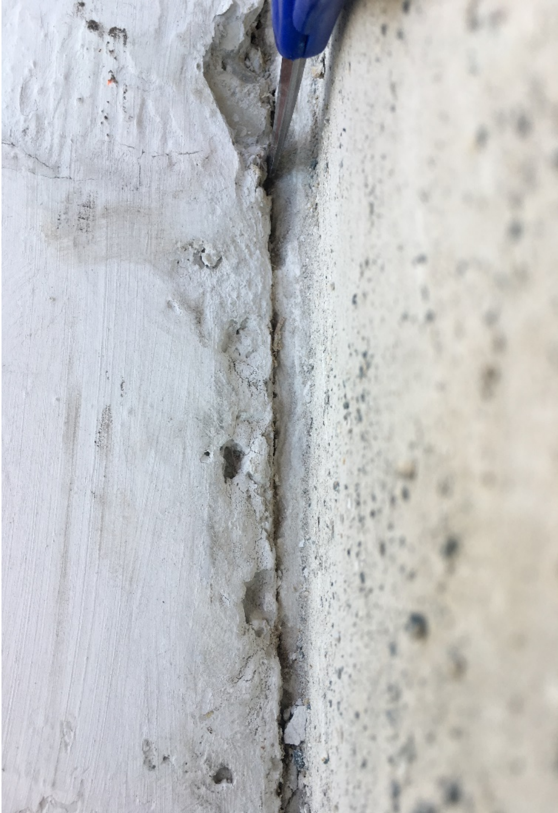
Figure 33 Cracks at the construction joint of the main span deck and diagonal 11 on 3/13/2018 by BPA
