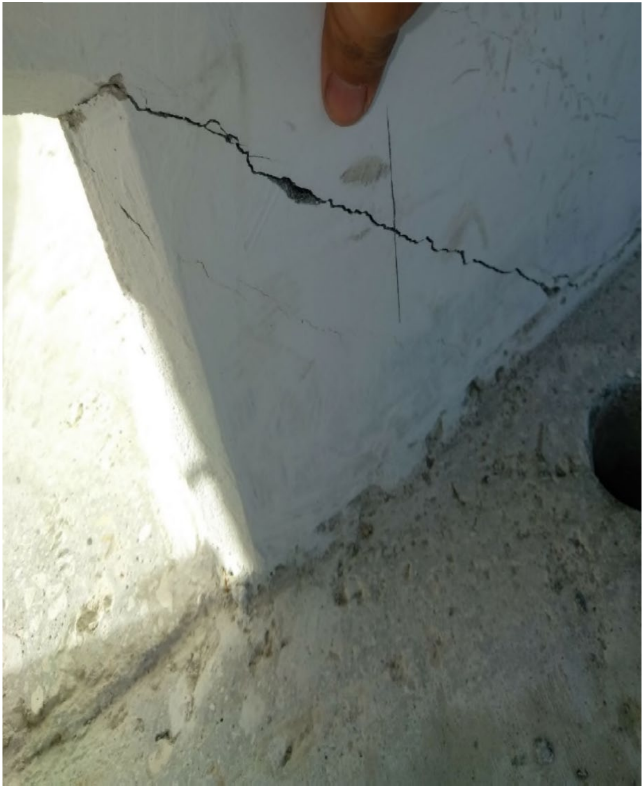
Figure 18 Photo #4 in 2/28/2018 E-mail from MCM to FIGG
