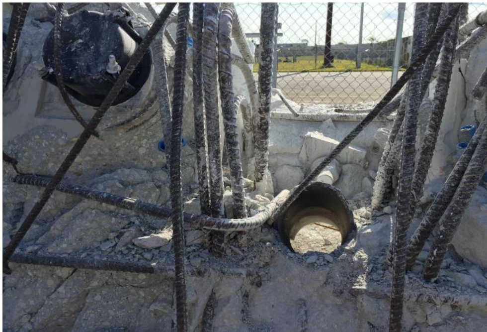
Figure 65 Punched hole in Diaphragm II at the time of the bridge collapse – from south looking towards north, April 9, 2018, by OSHA
