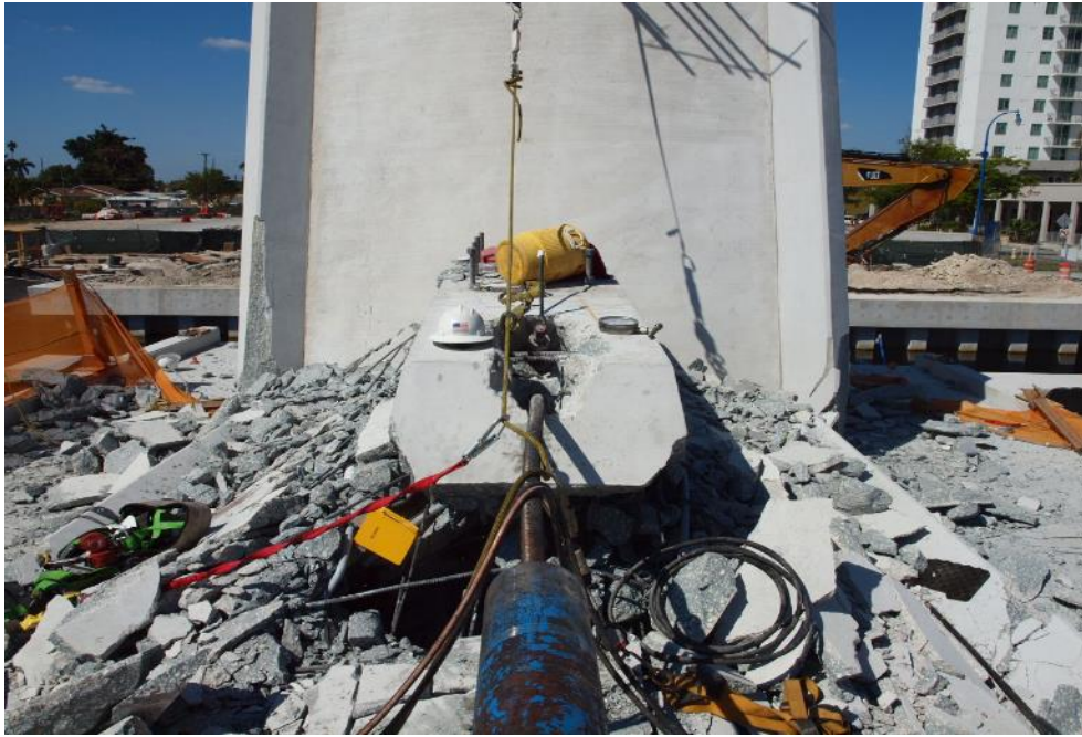
Figure 54 Northernmost blister and hydraulic jack attached to the lower PT bar of diagonal 11 after bridge collapse – front view, March 17, 2018 by OSHA
