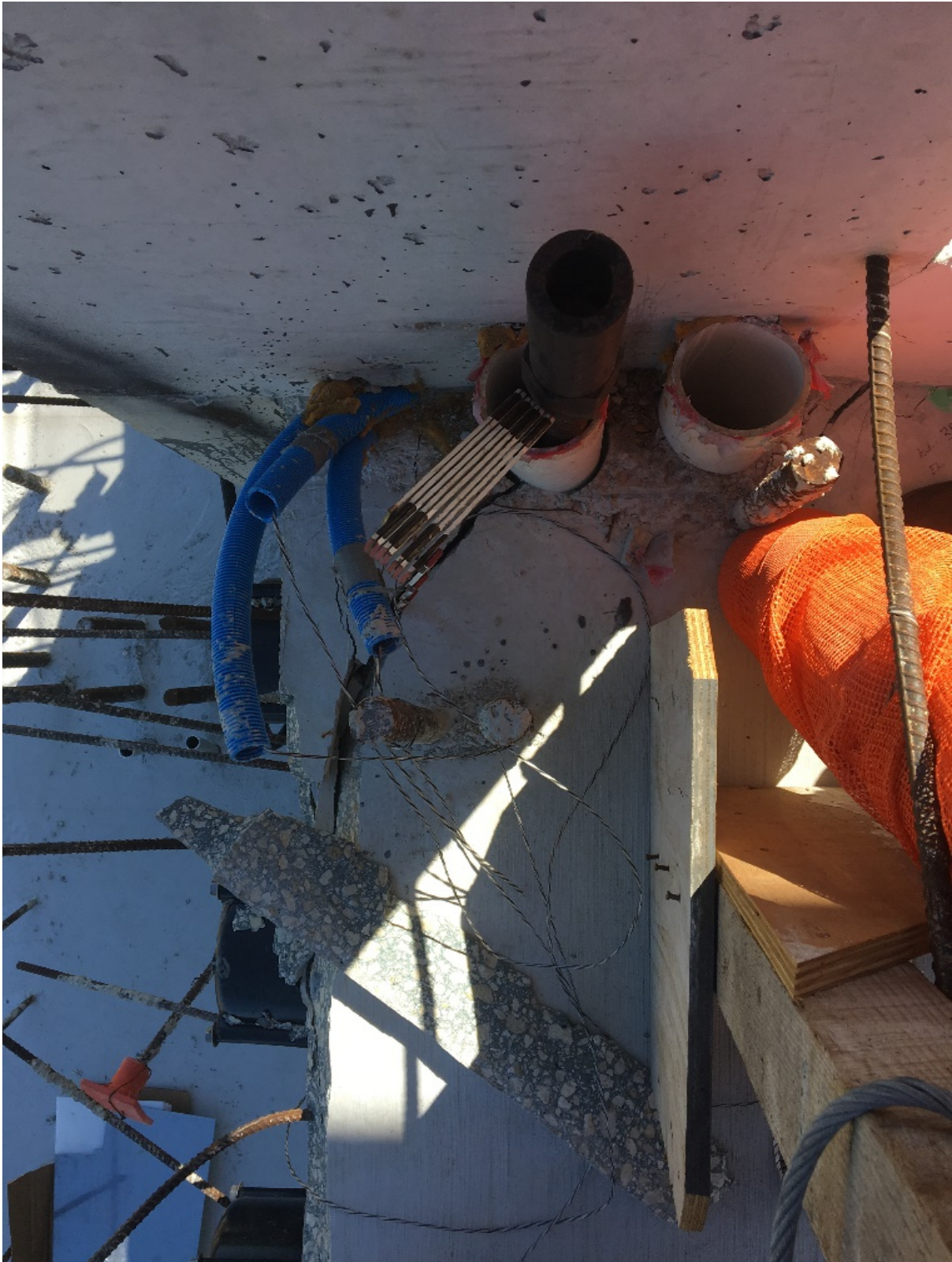
Figure 29 Close-up of cracks at the west side of diaphragm II on 3/13/2018, by BPA
