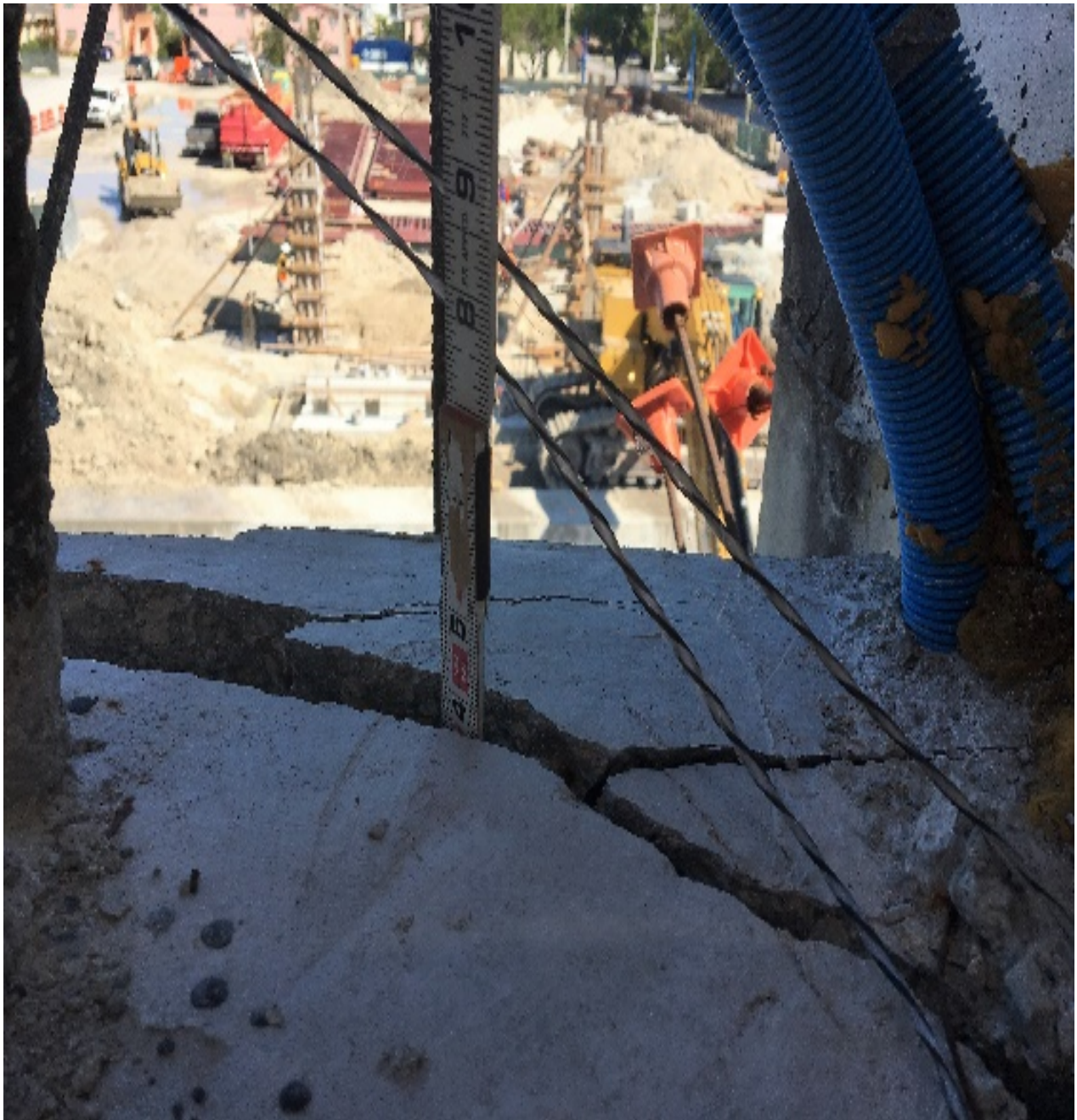
Figure 30 Notice the depth and width of diagonal cracks at the west side of diaphragm II on 3/14/2018 by BPA
