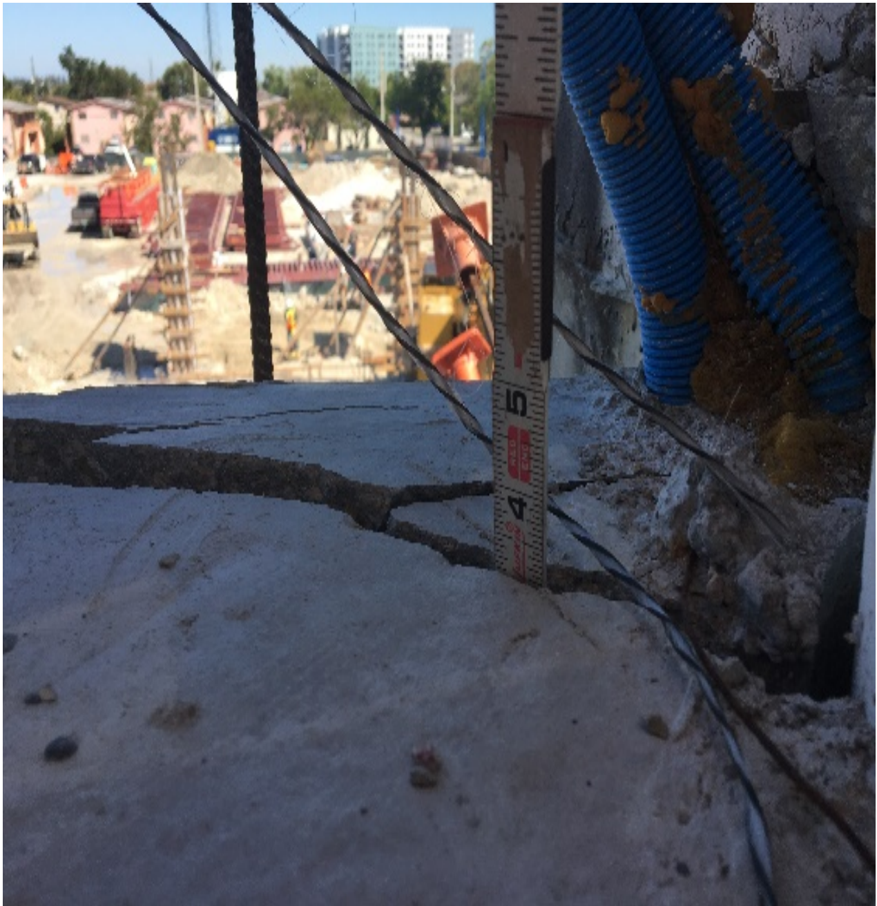
Figure 31 Notice the depth and width of cracks near column 12 at the west side of diaphragm II on 3/14/2018 by BPA
