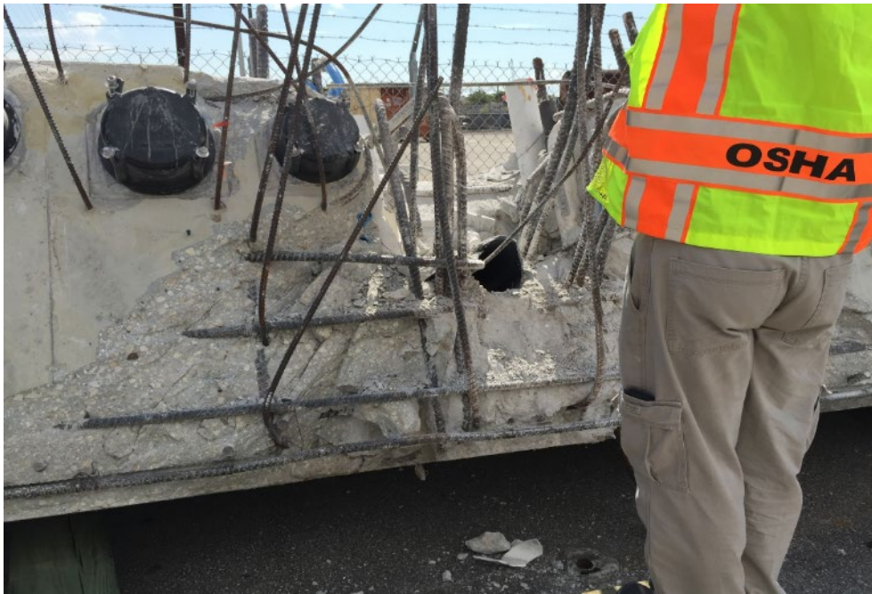
Figure 66 Punched hole in Diaphragm II at the time of the bridge collapse – from south looking towards north, April 9, 2018, by OSHA
