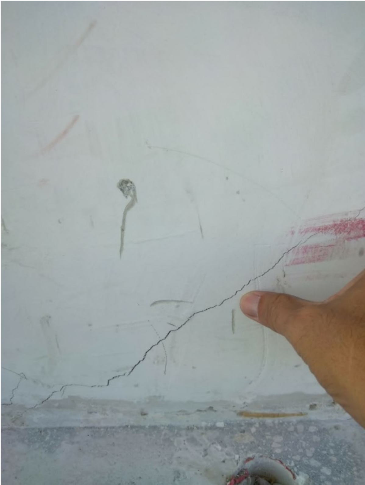
Figure 17 Photo #3 in 2/28/2018 E-mail from MCM to FIGG
