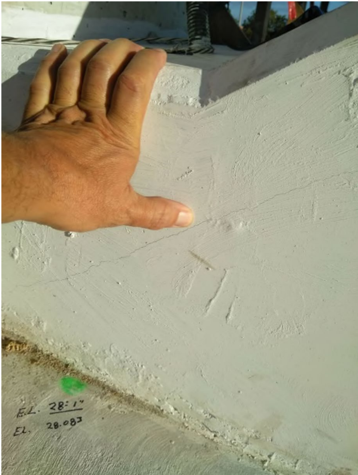
Figure 19 Photo #5 in 2/28/2018 E-mail from MCM to FIGG
