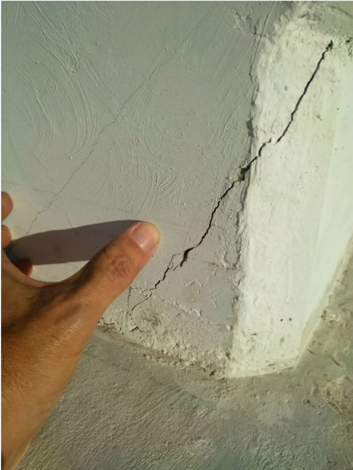
Figure 20 Photo #6 in 2/28/2018 E-mail from MCM to FIGG
