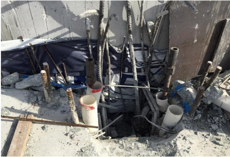
Figure 58 Concrete blow-out failure in Diaphragm II at the time of bridge collapse at the site looking north from south, March 21, 2018, by OSHA
