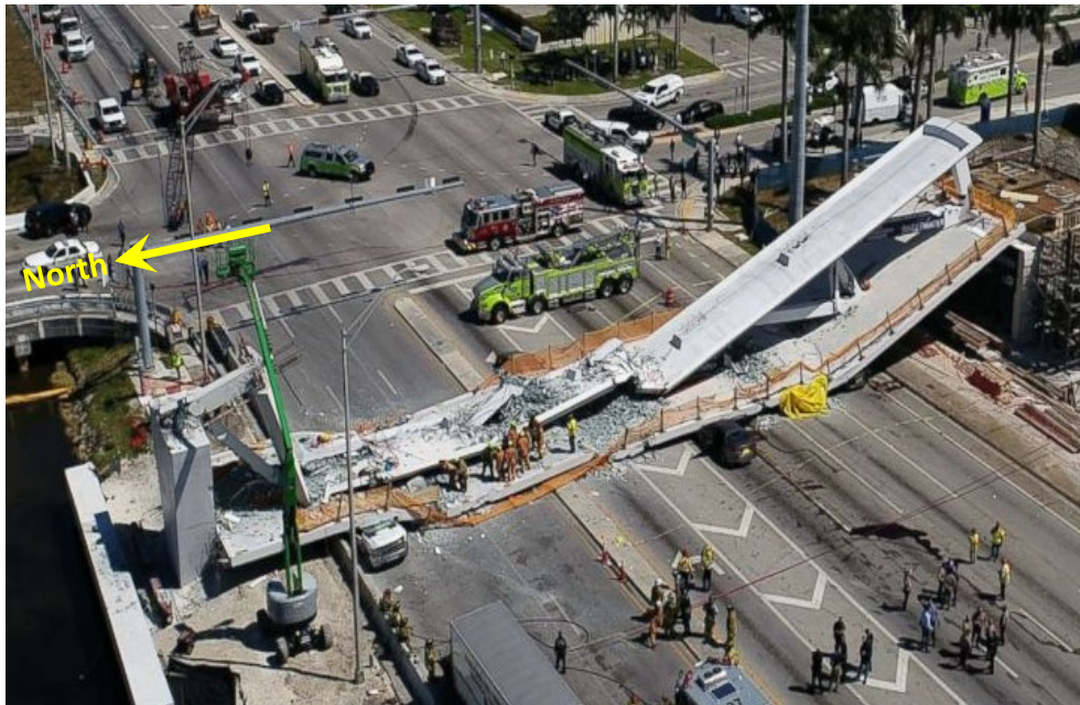
Figure 72 Aerial view of the collapsed bridge, March 15~18, 2018
