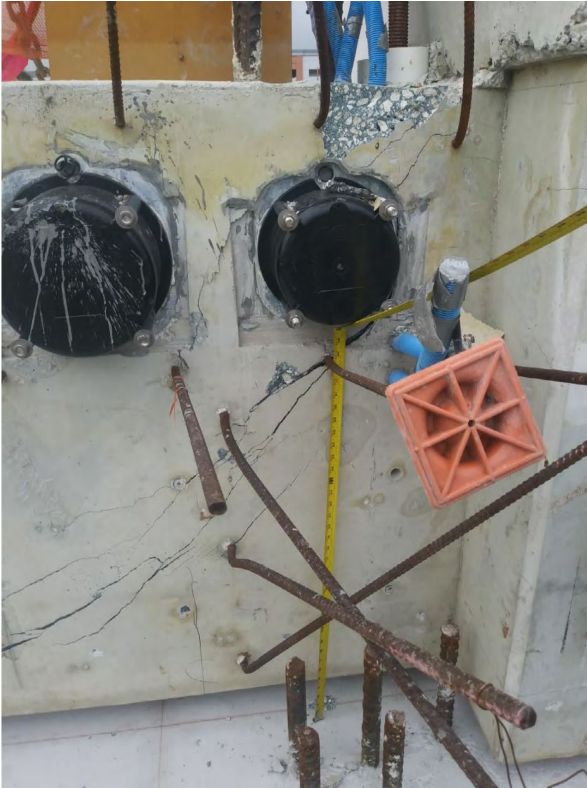
Figure 27 Cracks on the east side diaphragm II MCM email of 3/12/2018, by BPA – side face
