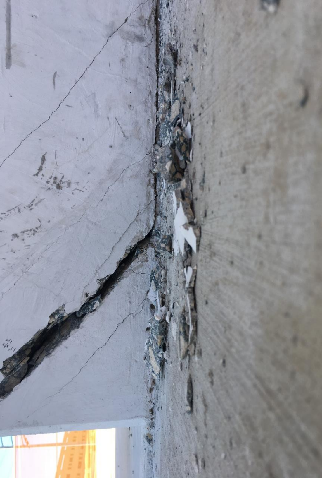
Figure 35 Cracks at the construction joint of the main span deck, diagonal 11 and the chamfer of diagonal 11 on 3/13/2018 by BPA
