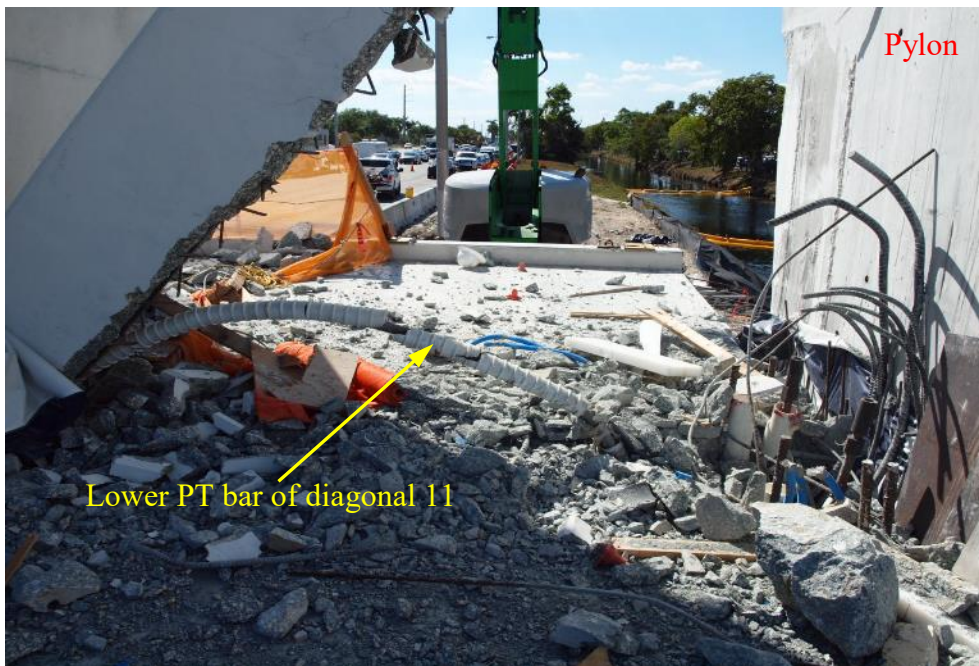
Figure 57 Lower PT separated from the diagonal 11 still embedded in diaphragm after bridge collapse, March 17, 2018 by OSHA
