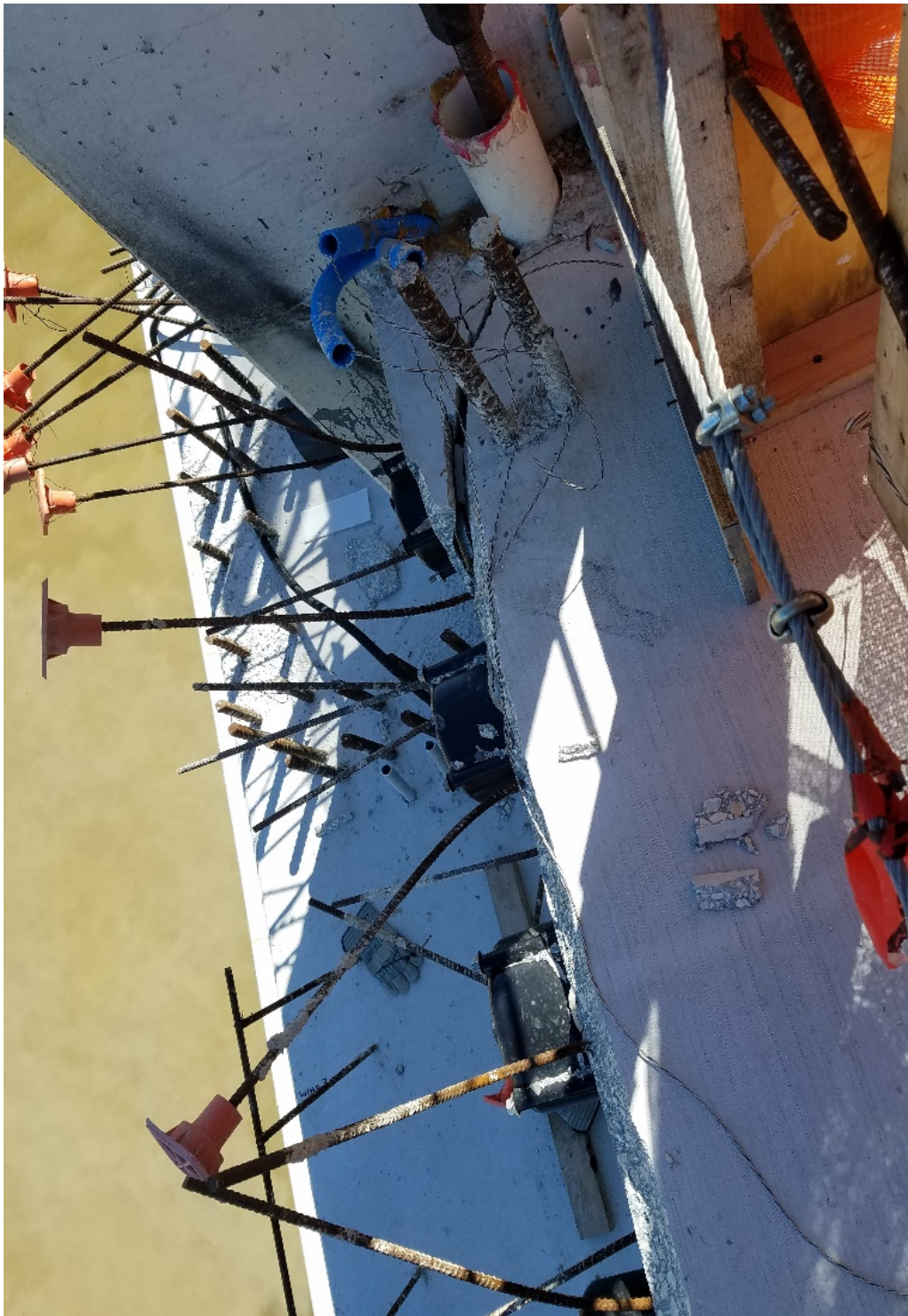
Figure 28 Diagonal cracks on the west side of diaphragm II on 3/13/2018, by BPA – top face
