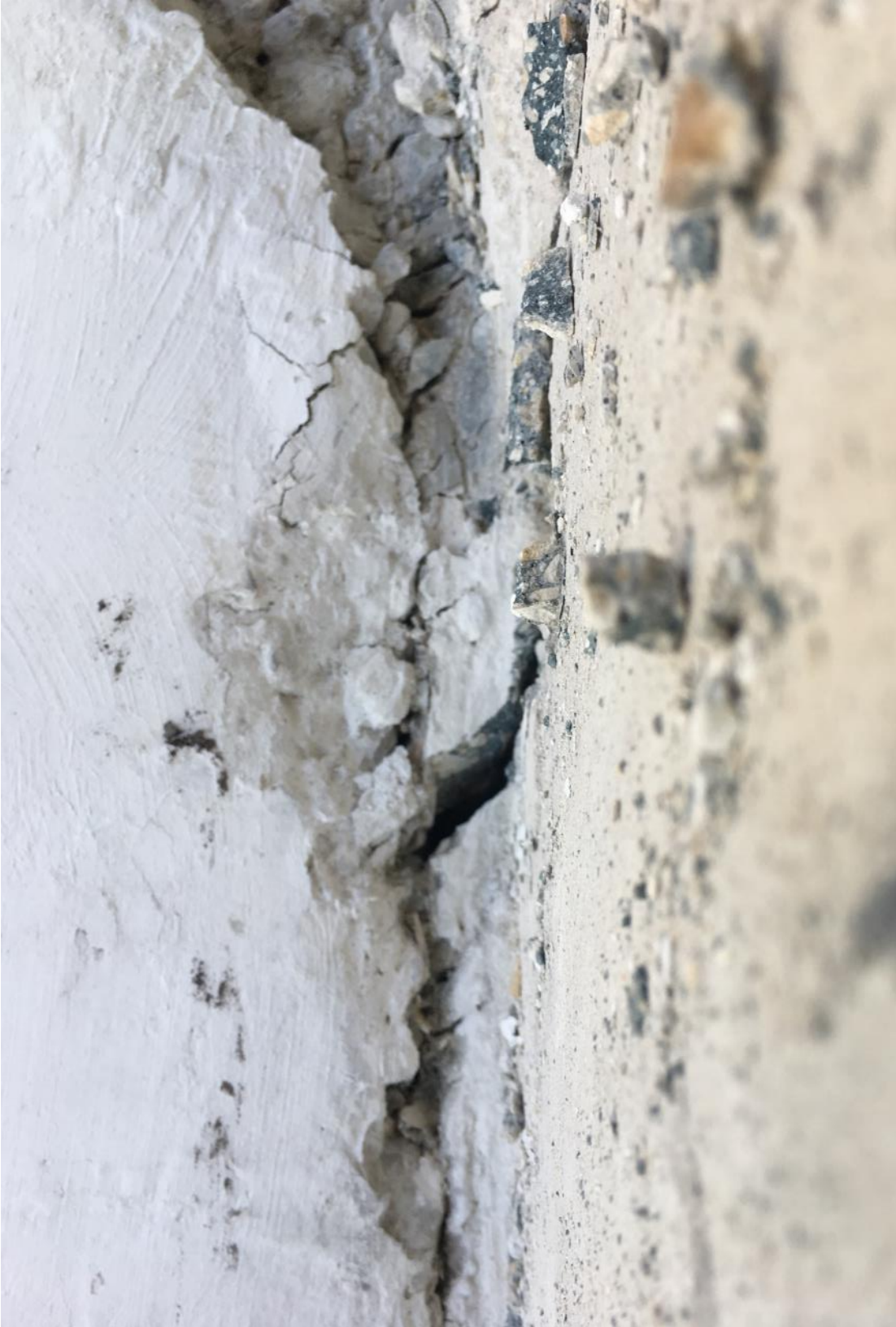
Figure 34 Cracks at the construction joint of the main span deck and diagonal 11 on 3/13/2018 by BPA
