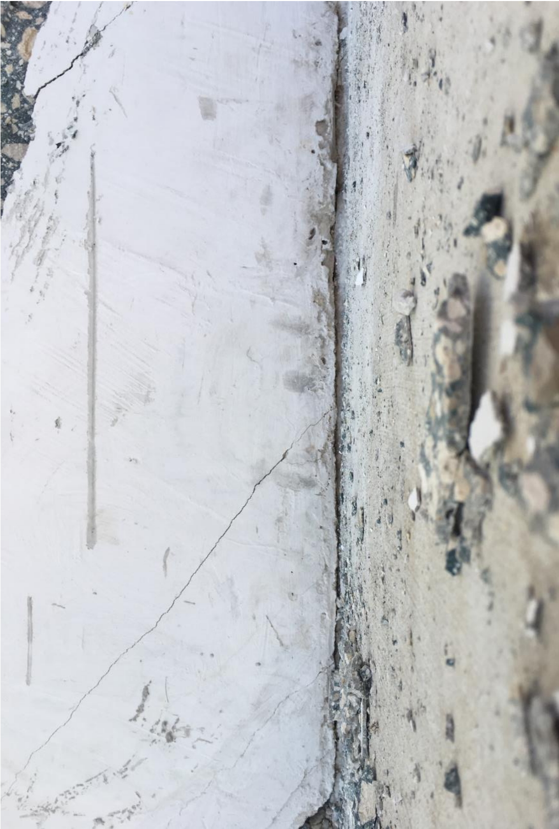
Figure 36 Cracks at the construction joint of the main span deck and diagonal 11 on 3/13/2018 by BPA
