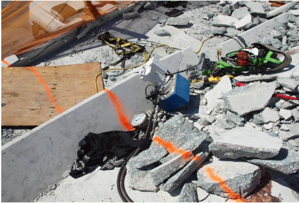
Figure 56 Hydraulic pump for post-tensioning after bridge collapse, March 17, 2018 by OSHA
