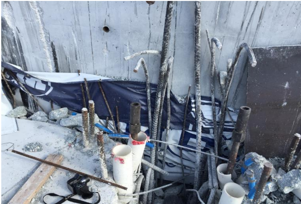
Figure 59 Concrete blow-out failure in Diaphragm II at the time of bridge collapse at the site looking north from south, March 21, 2018, by OSHA
