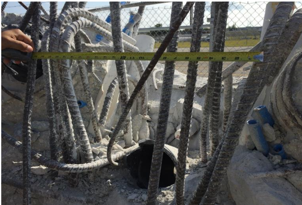
Figure 69 Punched hole in Diaphragm II at the time of the bridge collapse – from south looking towards north, April 9, 2018, by OSHA
