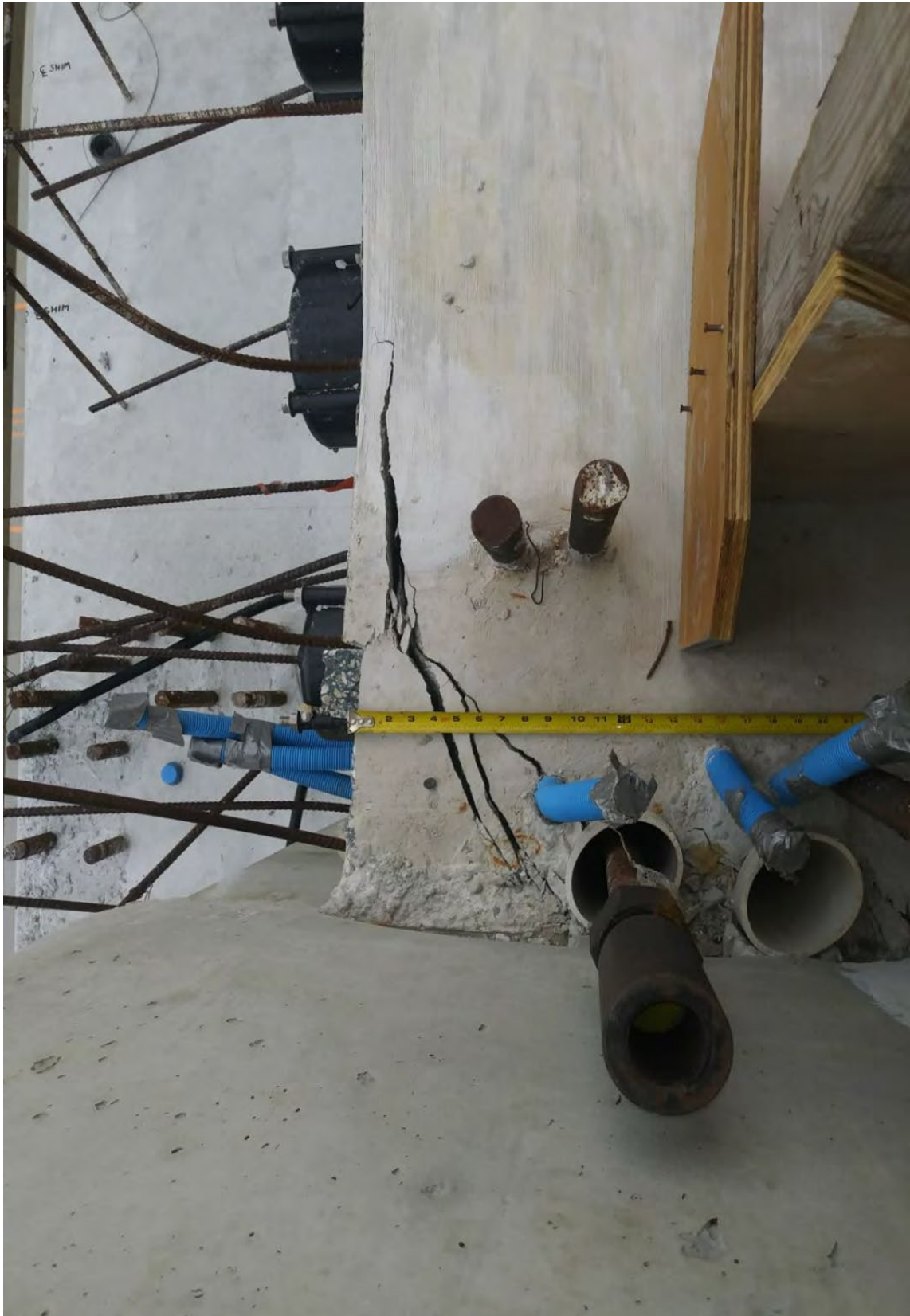
Figure 26 Cracks at the east side diaphragm II MCM email of 3/12/2018, by BPA – top face
