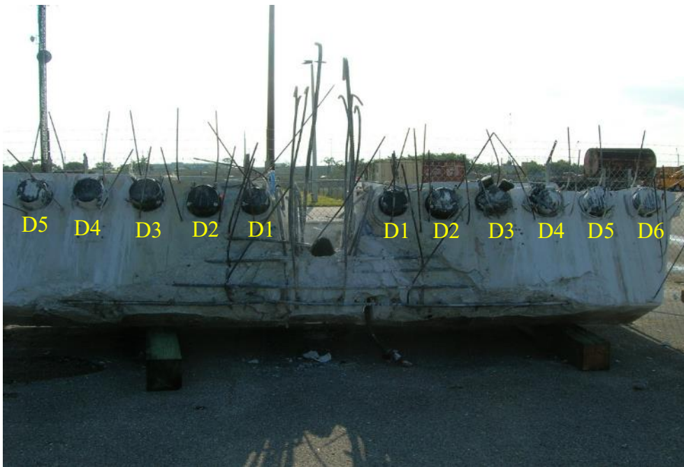
Figure 61 Remnants of diaphragm II at the time of the bridge collapse in the storage yard – looking north from south, April 9, 2018, by OSHA
