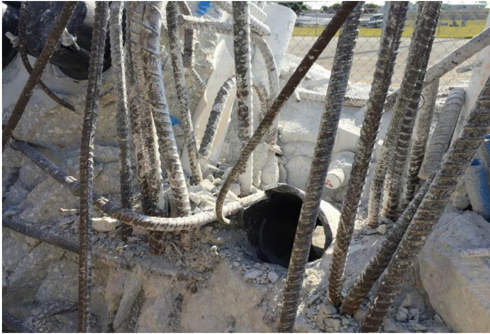
Figure 70 Punched hole in Diaphragm II at the time of the bridge collapse – from south looking towards north, April 9, 2018, by OSHA
