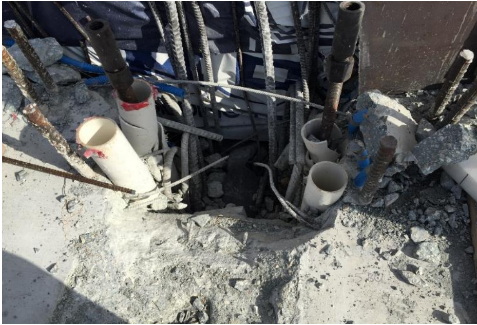
Figure 60 Concrete blow-out failure in Diaphragm II at the time of bridge collapse at the site looking north from south, March 21, 2018, by OSHA
