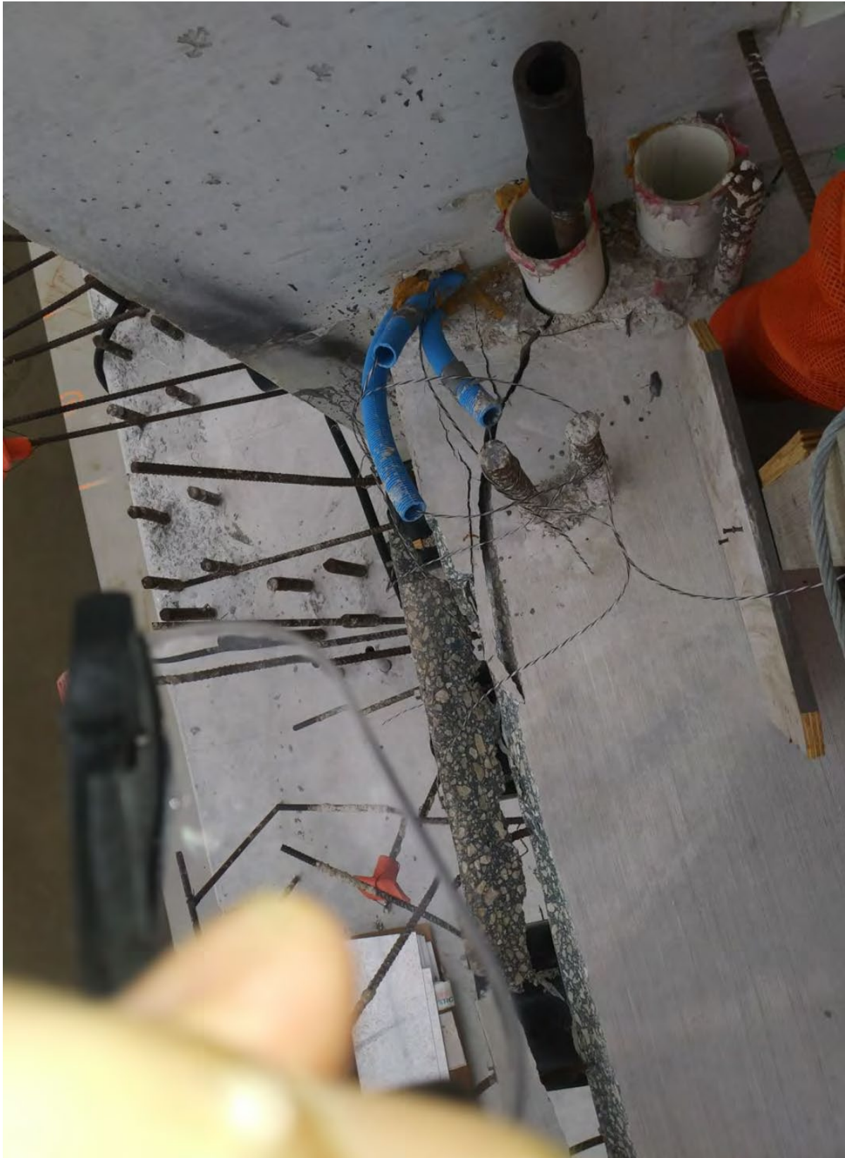
Figure 24 Cracks at the west side diaphragm II MCM email of 3/12/2018 – top face, by BPA.
