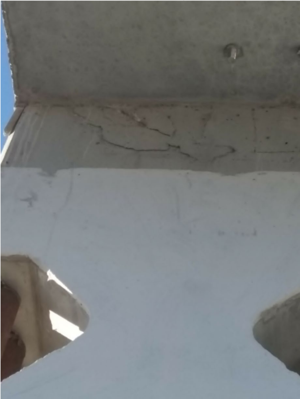
Figure 15 Photo #1 in 2/28/2018 E-mail from MCM to FIGG
