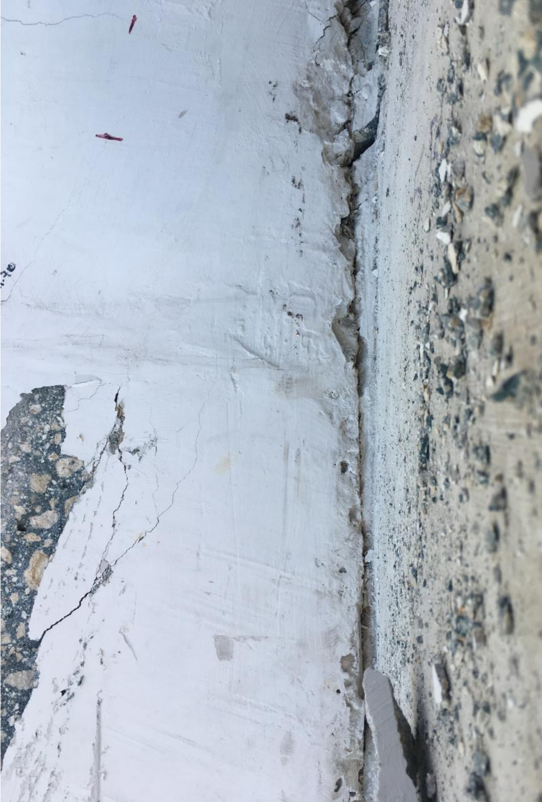
Figure 38 Cracks at the construction joint of the main span deck and diagonal 11 on 3/13/2018 by BPA
