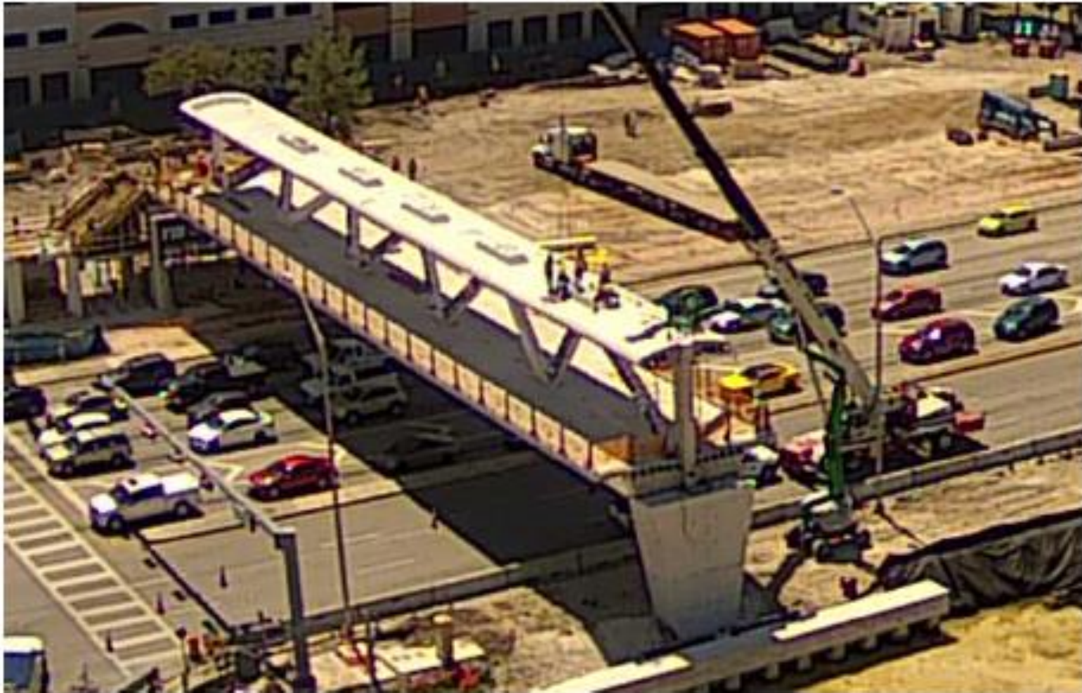
Figure 48 Bridge immediately prior to the collapse, March 15, 2018 – camera #2
