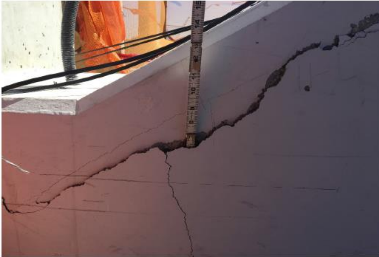
Figure 39 Close-up of longitudinal cracks in diagonal 11 on 3/14/2018 by BPA
