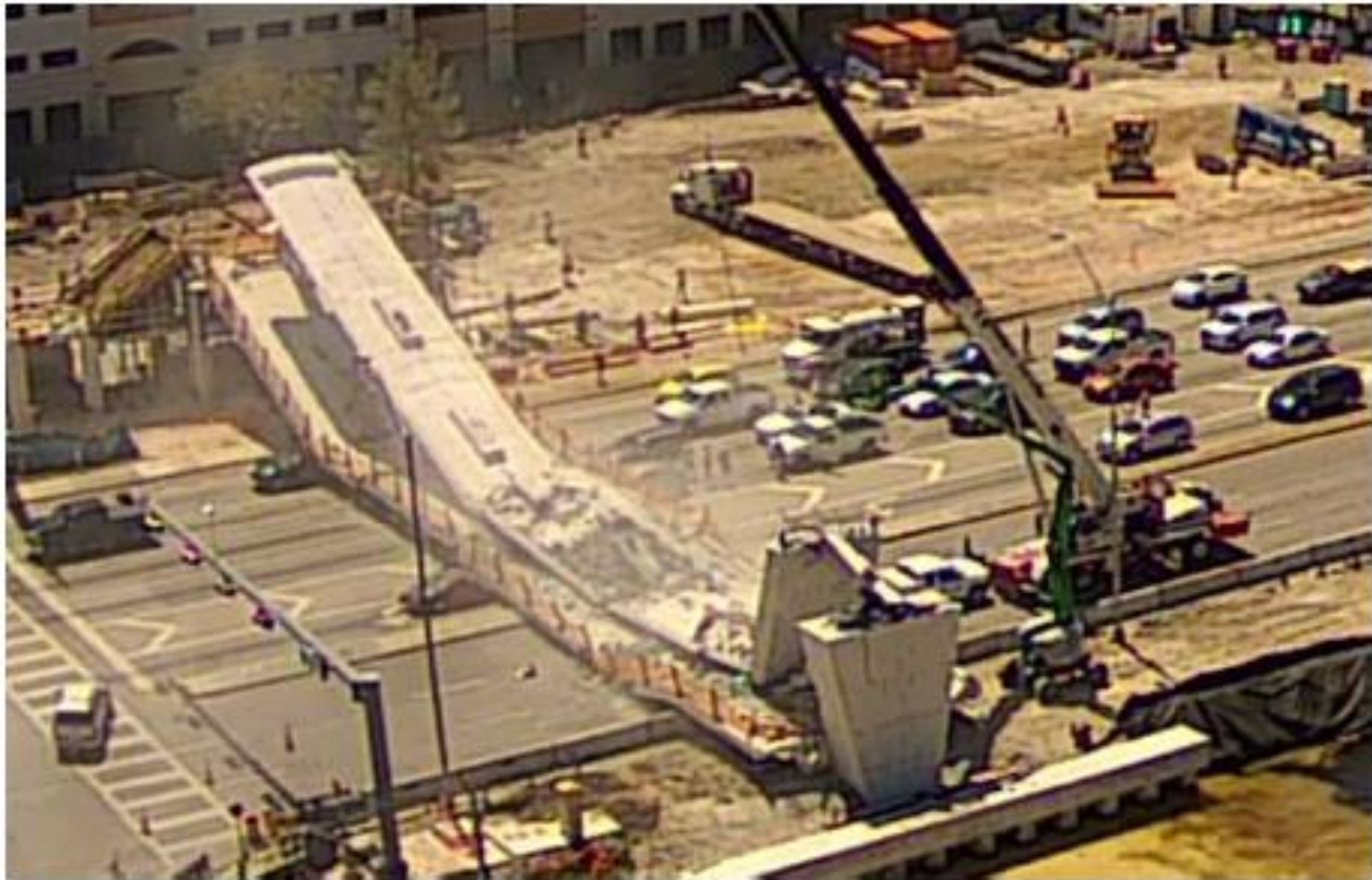
Figure 49 Bridge immediately after the collapse, March 15, 2018 – camera #2 Employees engaged in re-tensioning the PT bars in diagonal 11
